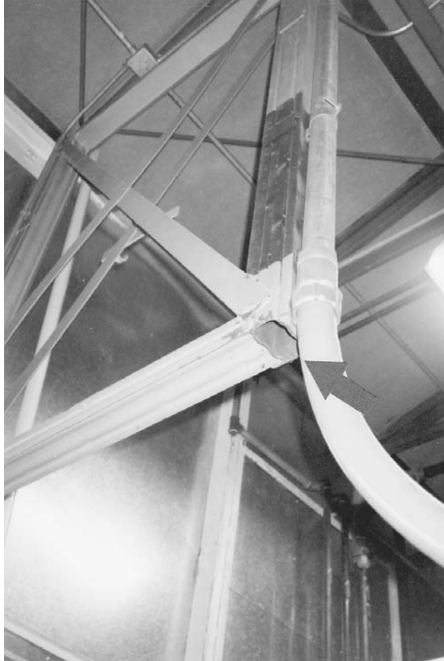
FIGURE 10.25 The bottom part of this interior wind-bracing bent was partly removed during previous alterations. This condition jeopardizes lateral-load resistance of the building.
